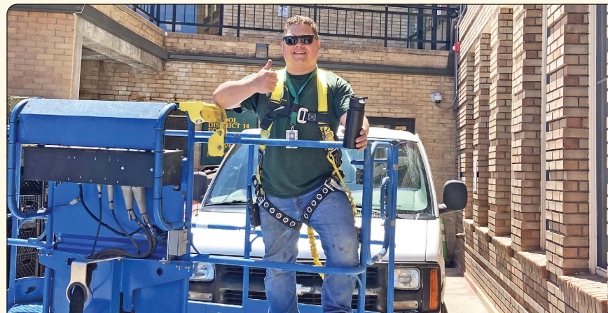
Buildings and Grounds Staff (Pete Sheloski, pictured) tackled the repair of the outside lights around Manitou Springs Elementary School!
